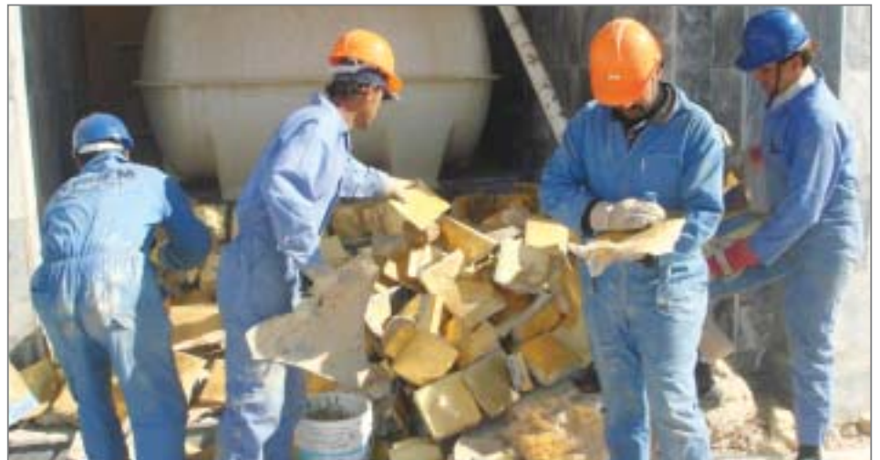
Iraqi workers collect gold plates which once covered the dome of the destroyed historic shrine of the Shiite Imam Al-Askari in Samarra at the start of reconstruction work on February 5, 2008.
